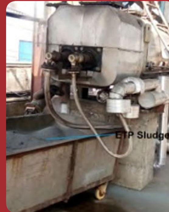
ETP Paddle dryer with dry sludge
